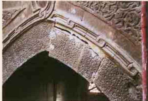
Seismic damage to decorative arches
