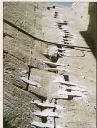
Vertical shear crack
