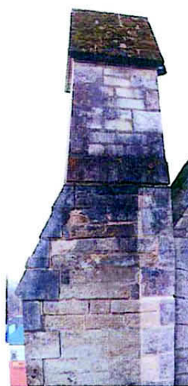
Ice damage and 'step' cracking
