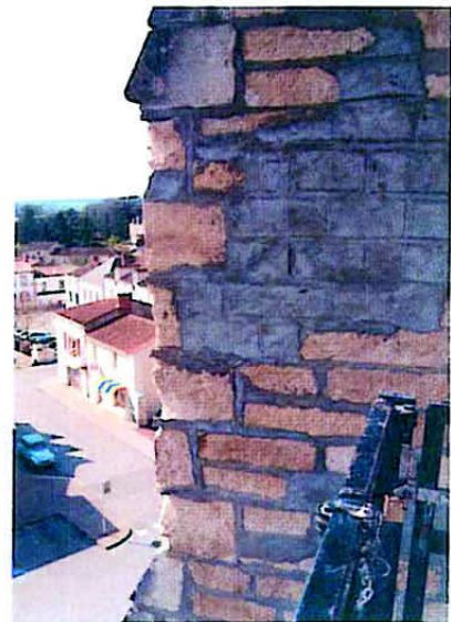
Degradation of limestone and old cement repairs
