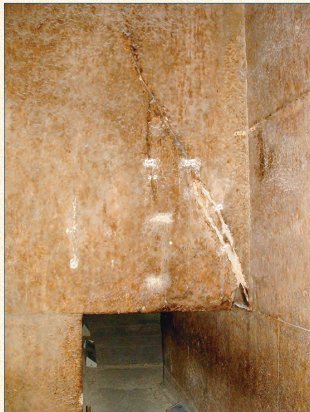
Front elevation of cracked beam
