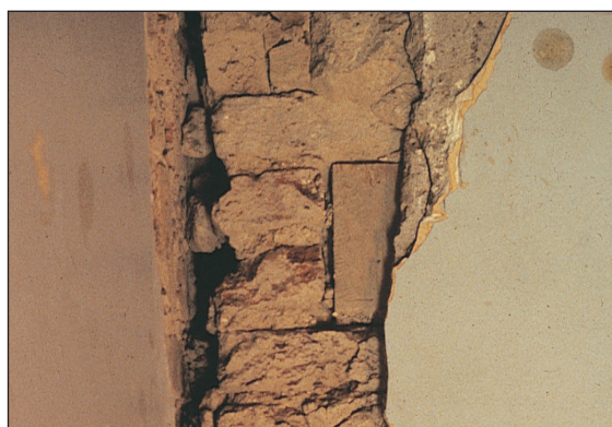
Internal damage of wooden beam
