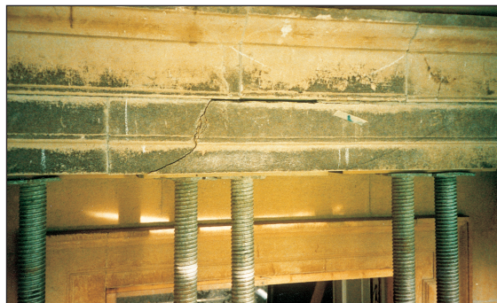
First sign of distressed beam
